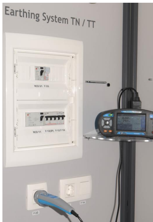
Figure 2-2: Measuring Z_{Line} in the Application Trainer with the schuko commander
