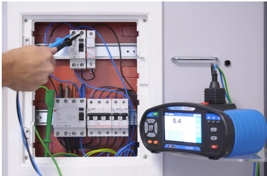
Figure 2-24: RCD measurement in Application Trainer’s switchboard with cables on the supply side
