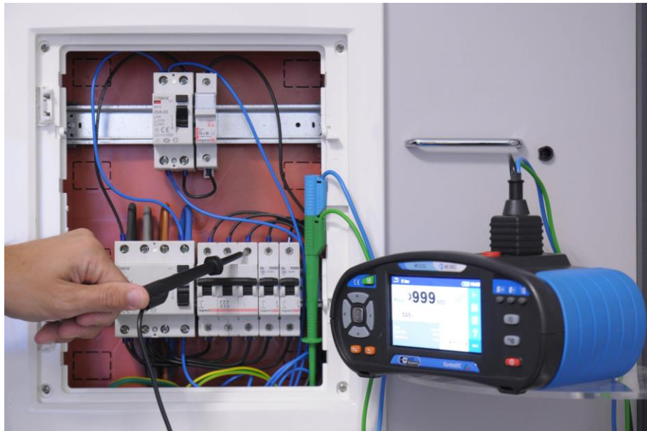
Figure 2-33: Insulation resistance measurement at the switchboard – all circuits on
