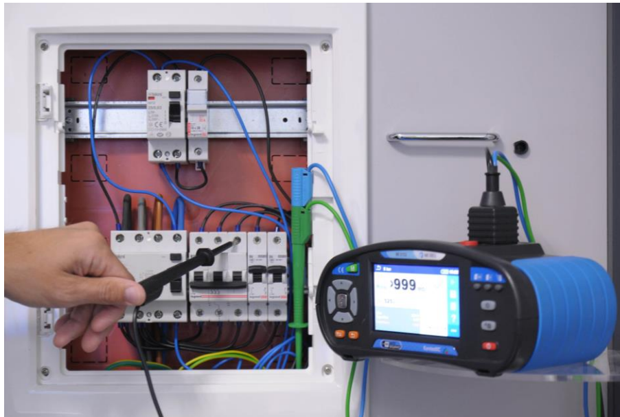
Figure 2-34: Insulation resistance measurement at the switchboard – disabling circuits during measurement
