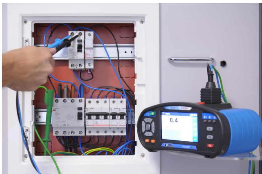
Figure 2-12: Measuring Z_{Loop} in Application Trainer's switchboard with cables on the supply side (before the RCD)
